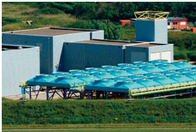
Cooling plant in Sangatte (FR)
