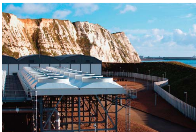
Cooling plant at Shakespeare Cliff (UK)
