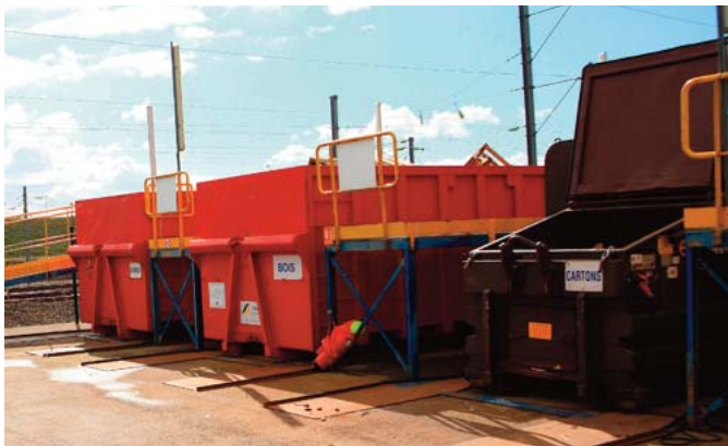
Waste collection plant on Eurotunnel Terminals: priority to waste sorting
